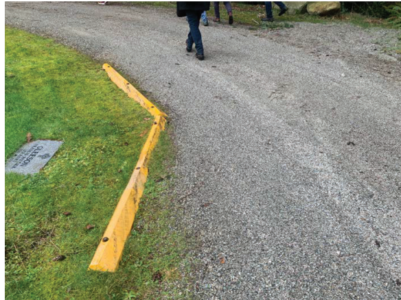
Figure 24: Existing curbing. Opportunity to enhance the cemetery appearance with asphalted driveways and concrete curbing.
