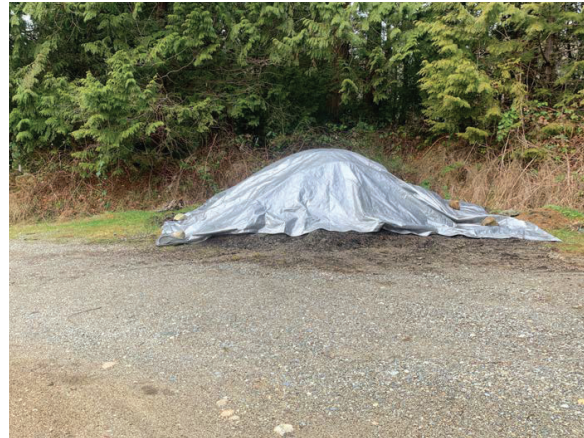
Figure 20: North west corner soil pile. Need to enhance aesthetic of bulk materials storage.
