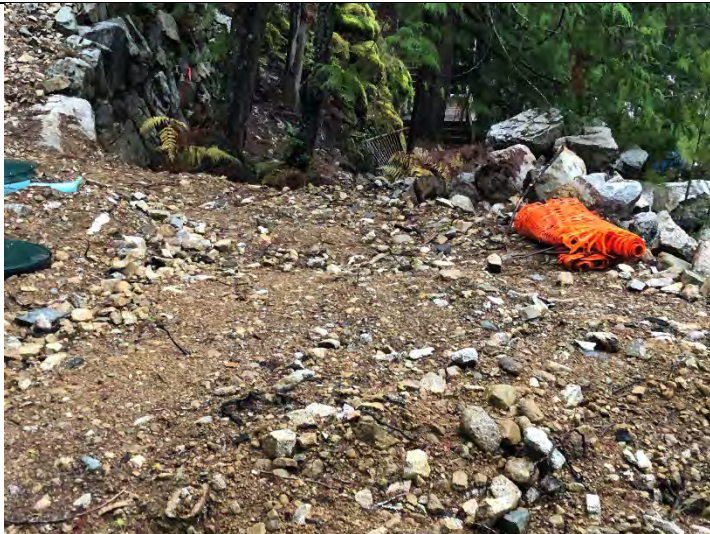
Photo 9: CIA disturbance in foreground, resulting from heavy equipment access for upland site preparation. . Viewing northeast. (Restoration Area- 2 – Fill).
