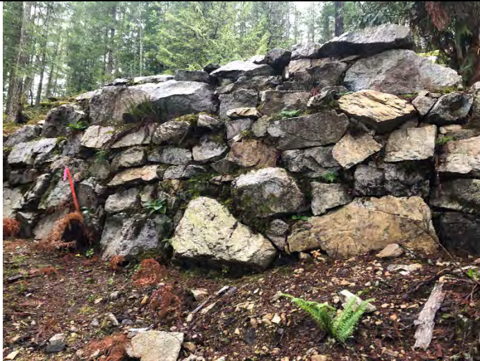
Photo 7: Rock wall constructed at 15m SPEA line. CIA disturbance in foreground. (Restoration Area - 1).
