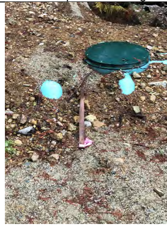
Photo 6. Upland building site, septic infrastructure near 13m variance line. (Restoration Area- 2 – Fill).
