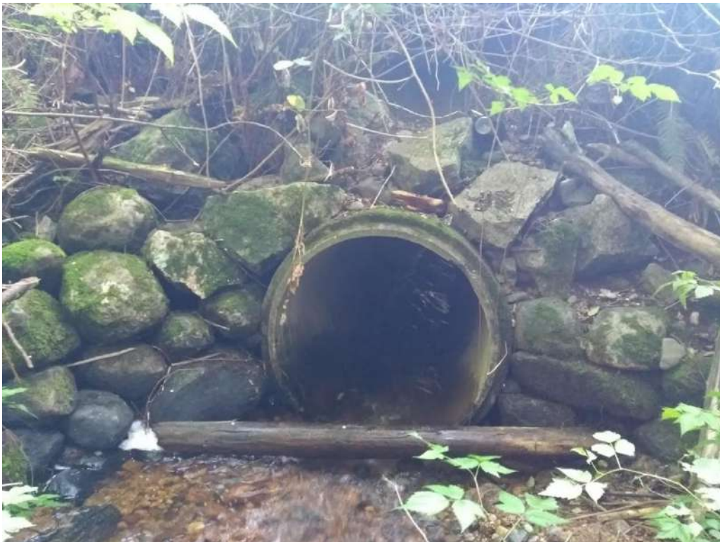
Photo 6: 1200mm diam. concrete culvert below Sunshine Coast Highway, approx. 25m downstream of bridge site.
