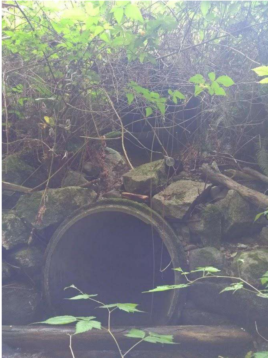
Photo 7: Same 1200mm diam. concrete culvert as previous photo but showing the 1200mm diam corrugated steel culvert stacked approx. 0.45m above (partially hidden by blackberry bush).
