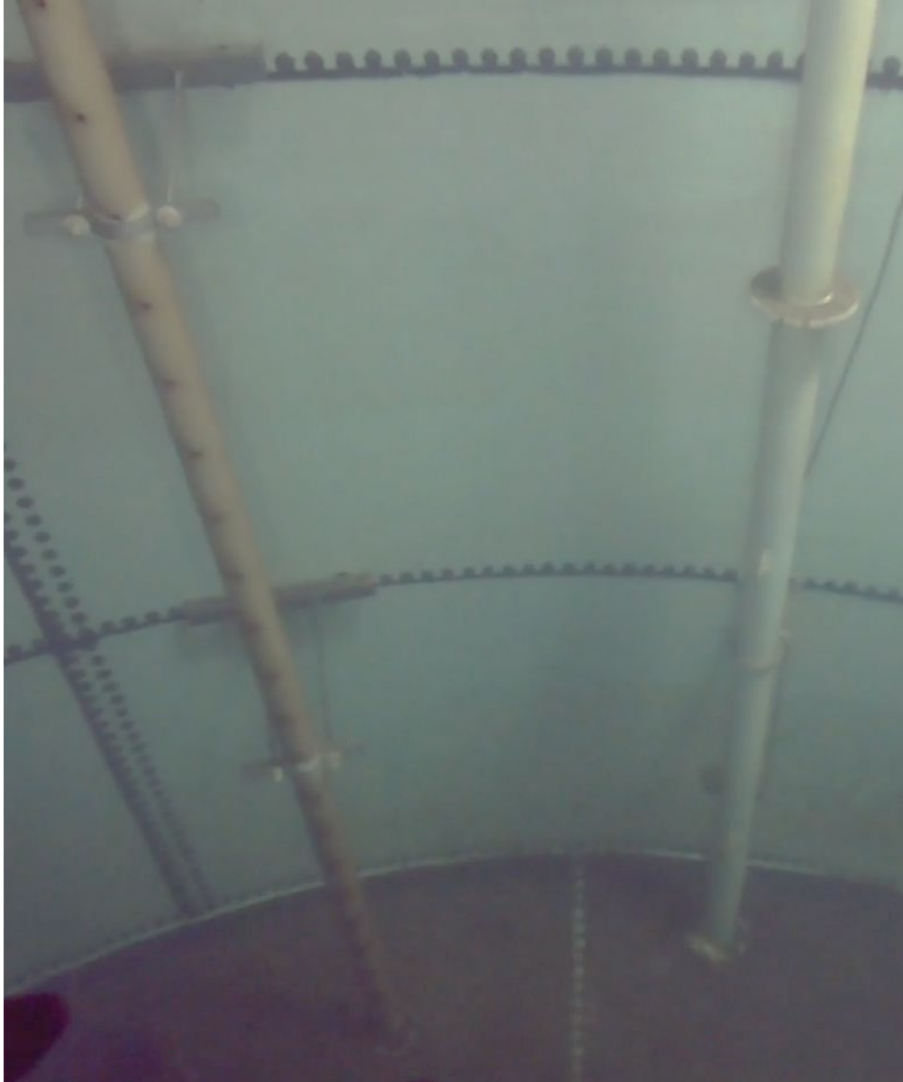
Image 1 - Overflow and Inlet pipes
