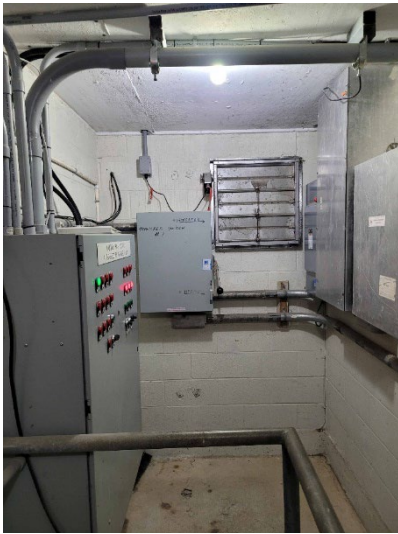
Photo 1 – Back wall. Design location of new ATS. Note approximately 64" from floor to bottom of powered ventilation louvre.
