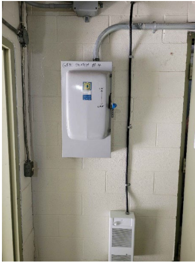
Photo 2 – Existing location of manual transfer switch. See markup below to consider this location as an alternative to the design location.
