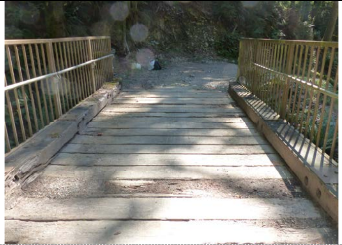
010 – Deterioration of Entire Timber Plank, View Looking East (D.1)
