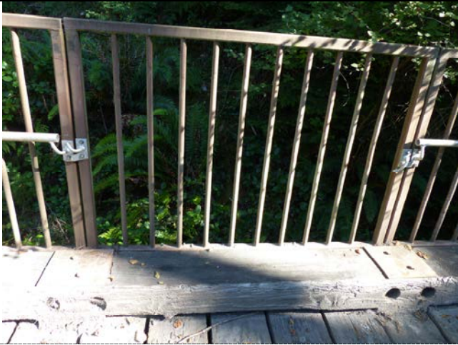
015 – Missing Railing - Appeared to be Torn off (D.6)
