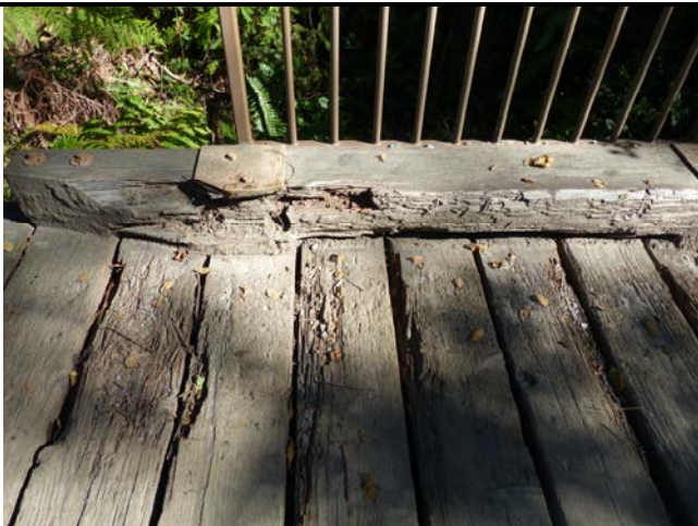
011 – Tread marks and Collision Damage at Bull Rail, NW corner of Bridge (D.2, D.4)
