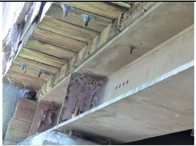
008 – Close-Up of Rusting Stiffeners, SW End of Bridge (C.3)
