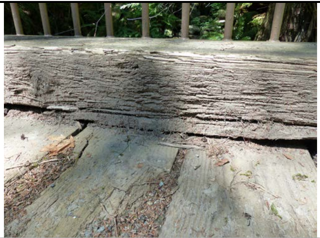
014 –Typical Timber Condition (D.4)
