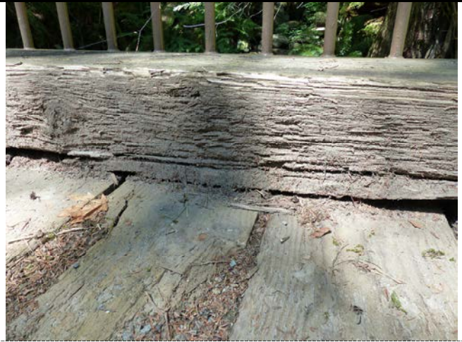
012 – Damaged Planking and Collision Damage on Bull Rail (D.2, D.4)
