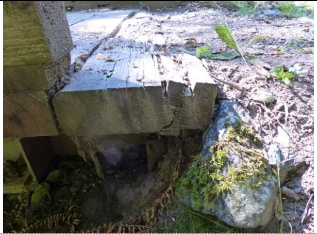
010 – Damaged Plank at NW Corner of Bridge (D.2)
