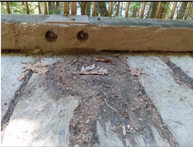
013 – Plank Deterioration and Isolated Rot in Bull Rail, Near SE corner of Bridge (D.2, D.4)
