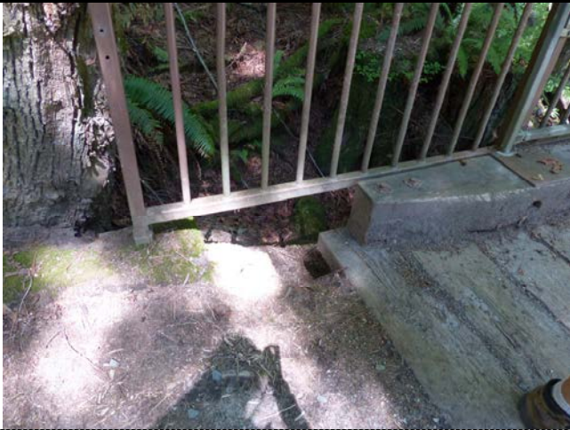
003 – Minor Erosion at NW Corner of Bridge (A.2)
