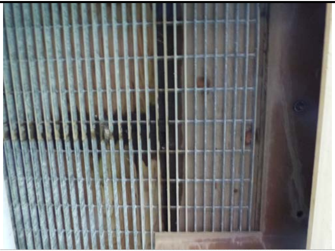
008 – Plywood between Steel Grating and Timber Planking (D.1)
