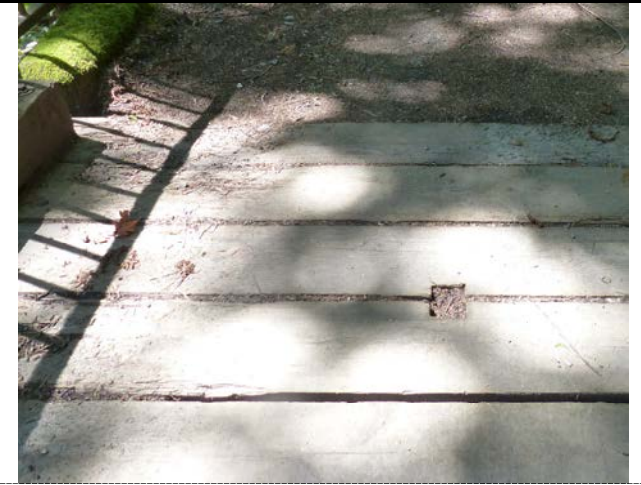
011 – Tread marks on Planking, SW corner of Bridge (D.2)
