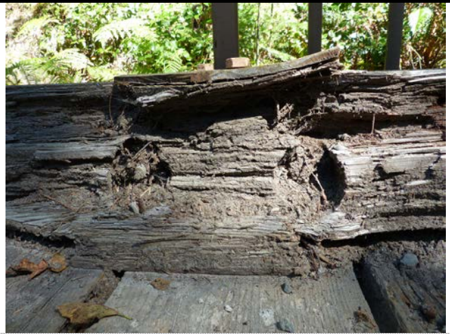
014 - Close-Up of Collision Damage at Bull Rail, NW Corner of Bridge (D.4)
