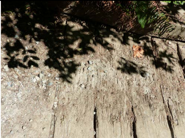
011 – Tread marks on Planking, NW corner of Bridge (D.2)
