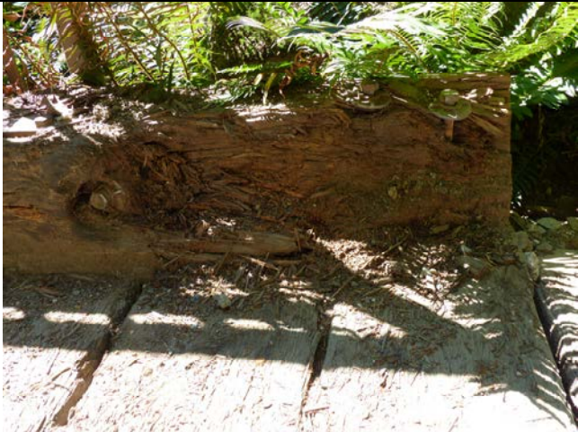
015 - Close-Up of Collision Damage at Bull Rail, SW Corner of Bridge (D.4)
