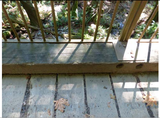
010 – Accumulation of Soil and Gravel between Planks and Wanes at Bull Rail (D.2, D.4)
