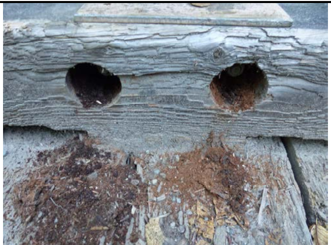
012 – Rotted Wood from Bolt Holes in Bull Rail (D.4)
