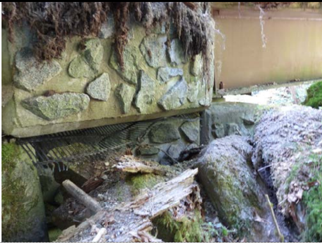
003 – Exposed Geotextile at Lock Block, West End of Bridge (B.1)
