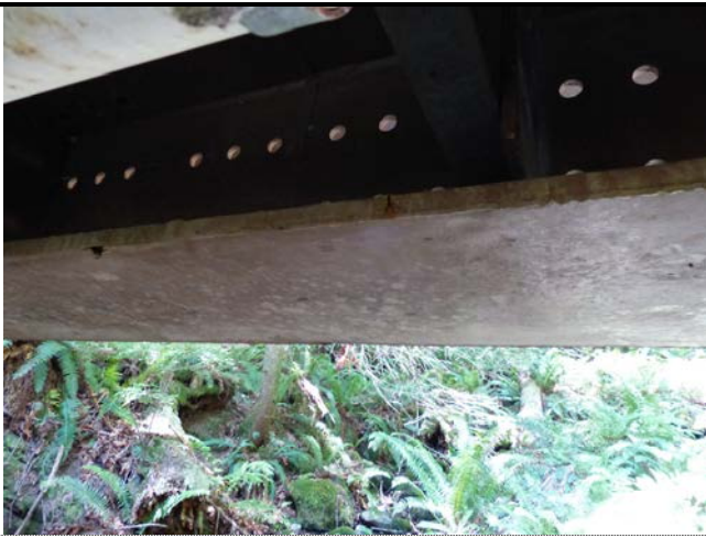
007 – Close-Up of Rusting Steel Girder, South side of Bridge (C.3)
