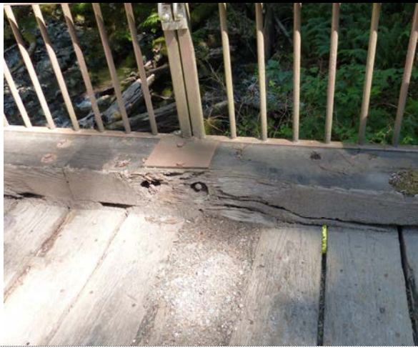
013 – Collision Damage at Bolt Holes in Bull Rail (D.4)
