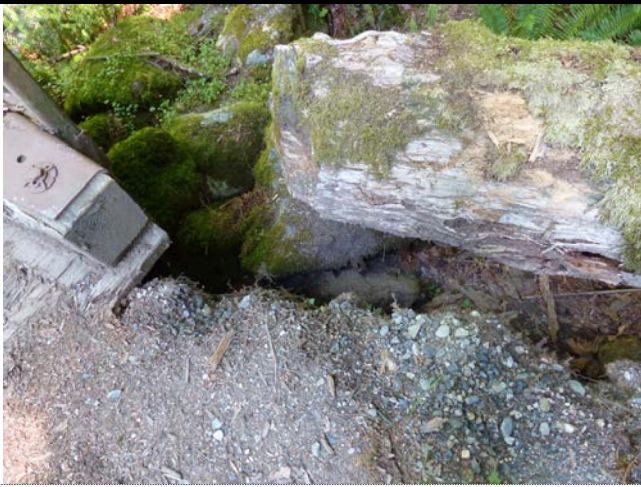
001 – Erosion at NE Corner of Bridge (A.2)
