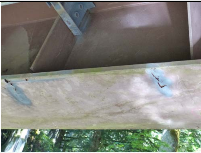
007 – Localized Scaling at Steel Girder, at East end of North side of Bridge (C.3)
