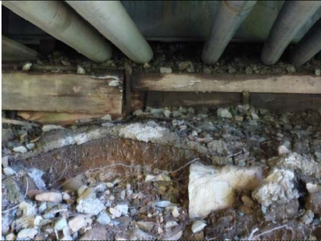
003 – Close-up of Foundation at East End of Bridge, Damp and Rotting Timber Sill (B.1)
