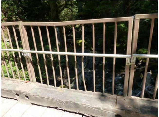
016 – Damaged Guardrail (D.6)
