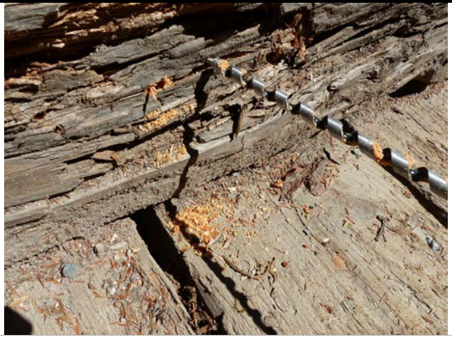
014 – Drill Hole at Rotting Bull Rail and Typical Timber Condition (D.4)
