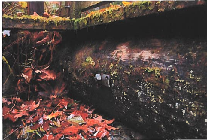
Photo 4 Vine Brook Bridge. South end of East stringer showing the end of the cross bar between the logs.
