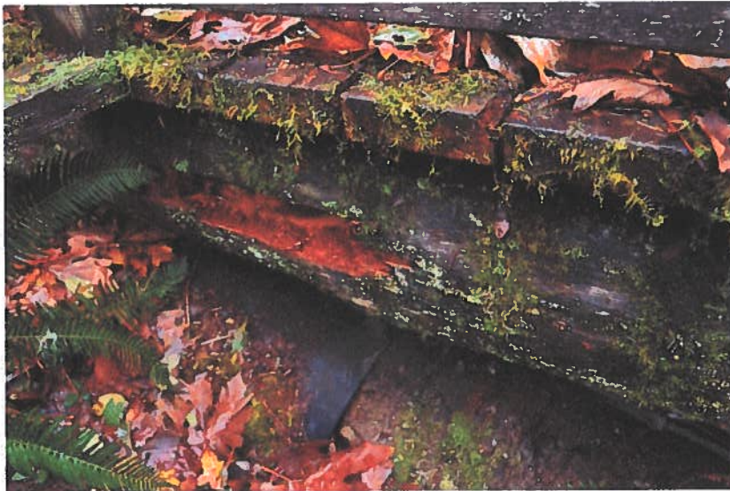
Photo3 Vine Brook Bridge. North end of West stringer log showing much deterioration.
