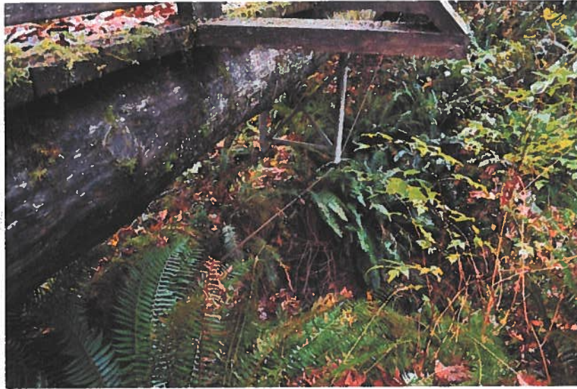
Photo 2 Vine Brook Bridge showing stringers supported at mid-span on steel frame and tension cables.
