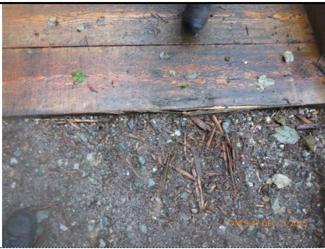
007 – Wearing at Planking, W Approach (D.2)
