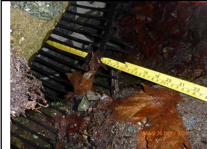
003 – Exposed Geotextile at Lock Block at NE Abutment -- Note approx. 200mm lock block displacement (B.1)
