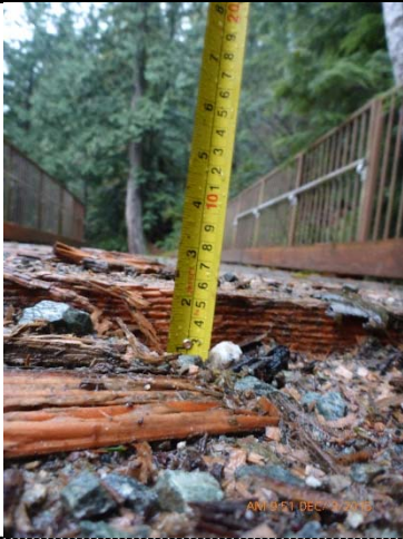
009 – East Approach Deck Elevation 55mm above Roadway Grade – Note wearing at planking (E.2)
