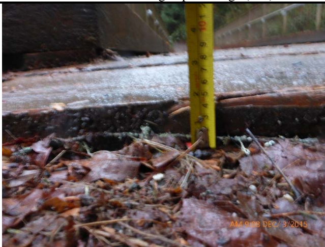
011 – East Approach Deck Elevation 45mm above Roadway Grade (E.2)
