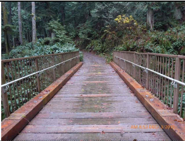
007 – View of General Condition of Bridge Deck & Curb Rails (D)
