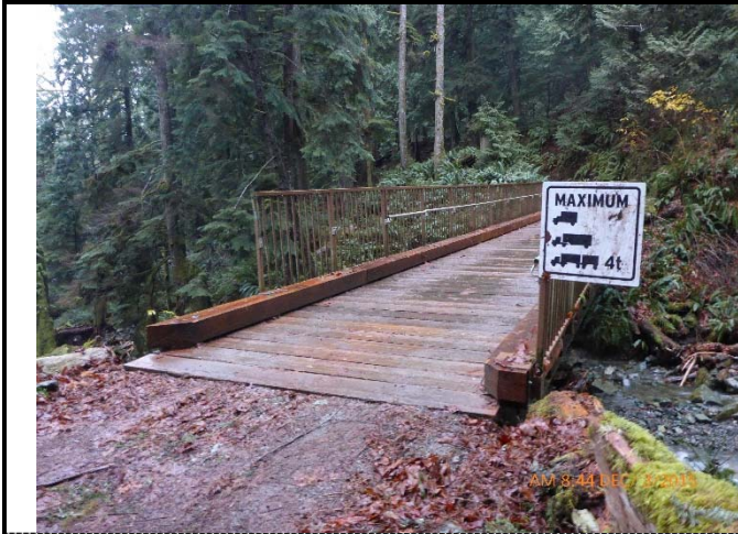
001 – View of Bridge from East Approach – Note missing guardrail and handrails at SE corner
