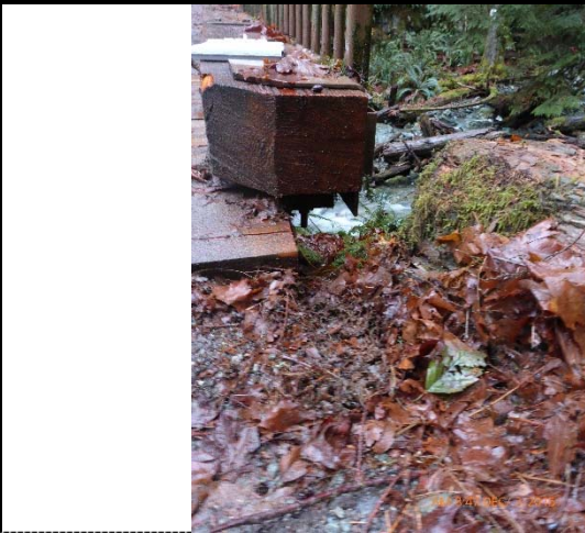
002 – Erosion at NE Corner of Bridge (A.2)
