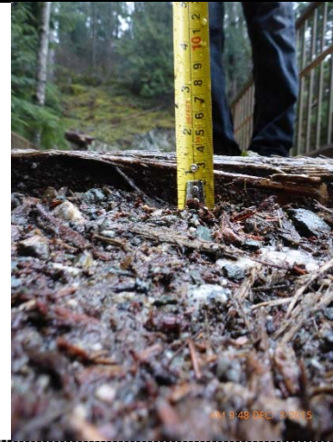
010 – West Approach Deck Elevation 35mm above Roadway Grade – Note wearing at planking (E.2)
