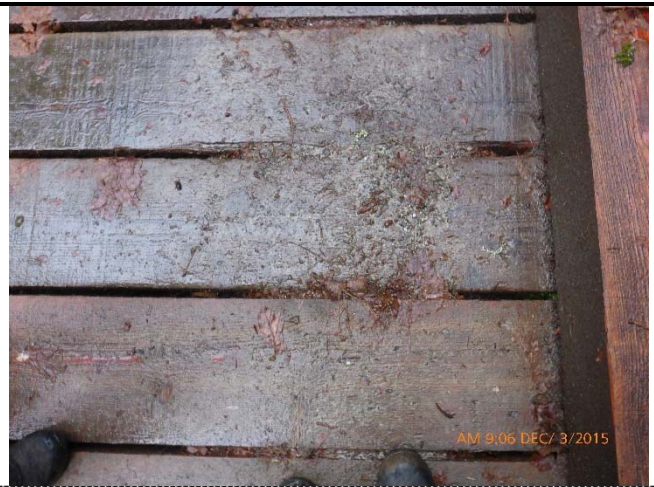
008 – Debris Accumulation Between Planks (D.1)
