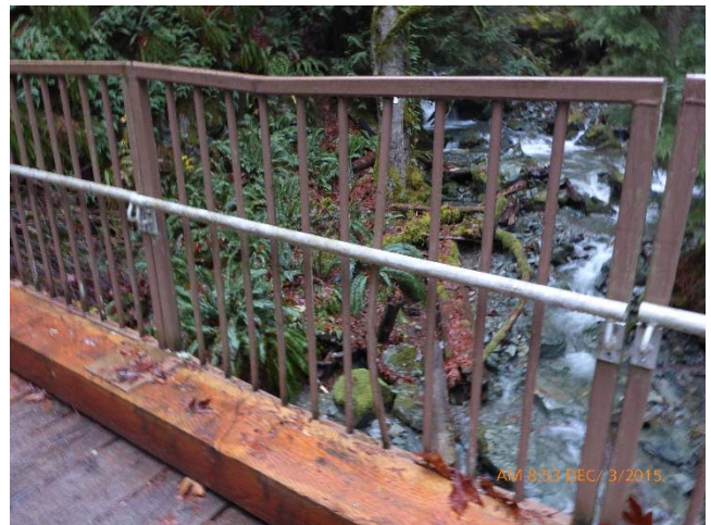
010 – Re-Used Guard Rail with Collision Damage near NE Corner of Bridge (D.6)
