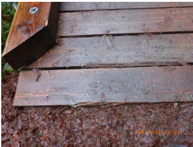
009 – SE Corner of Bridge, Repaired – Note minor wearing at plank edge (D.2)
