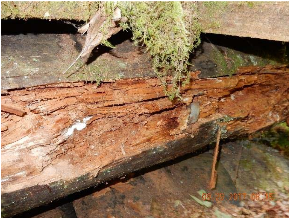
P10 – Northwest corner of the bridge, log is breaking apart (DSCN9856.jpg)
