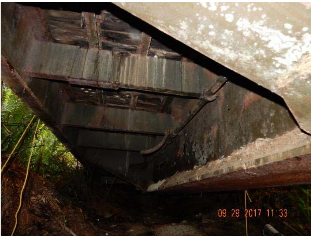
P14 – East side of the bridge, looking at three floor beams in between diaphragms (DSCN9969.jpg)
