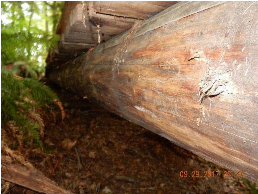
P11 – East side of the bridge (detail view of the log) (DSCN9882.jpg)
