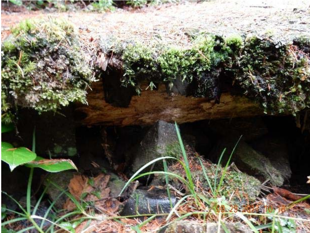
P05 – West side of the bridge, the entire deck is collapsing on rocks below it (DSCN9929.jpg)
