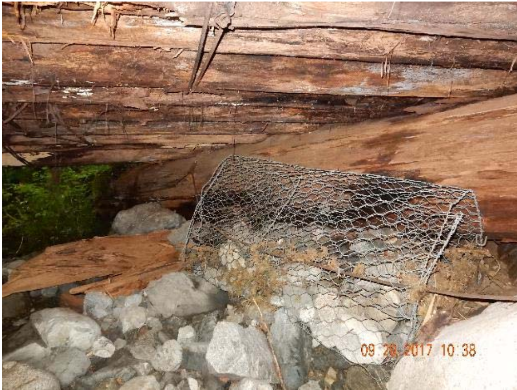
P09 – North abutment, gabion basket has fallen apart (DSCN9942.jpg)
