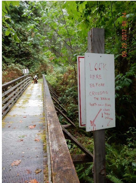
P07 – Sign at northwest corner of the bridge says, “Look here before crossing the bridge with your quad, check bridge stringer” (DSCN9853.jpg)
