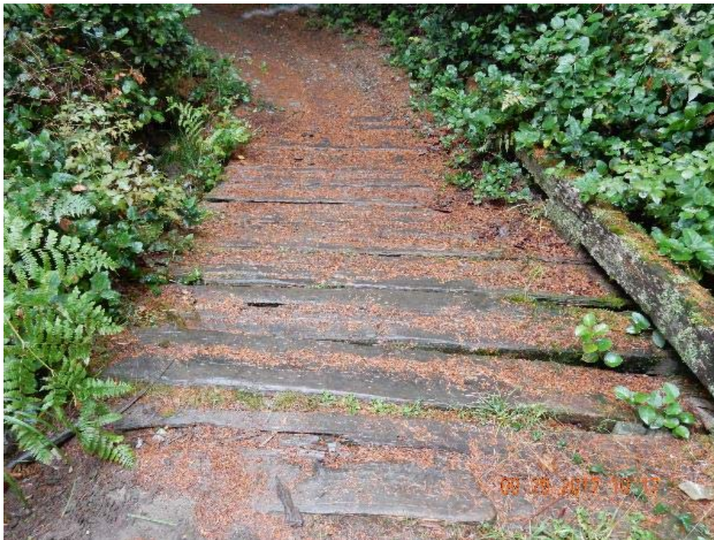
P02 – Overall decking, deck is in poor condition (DSCN9925.jpg)
