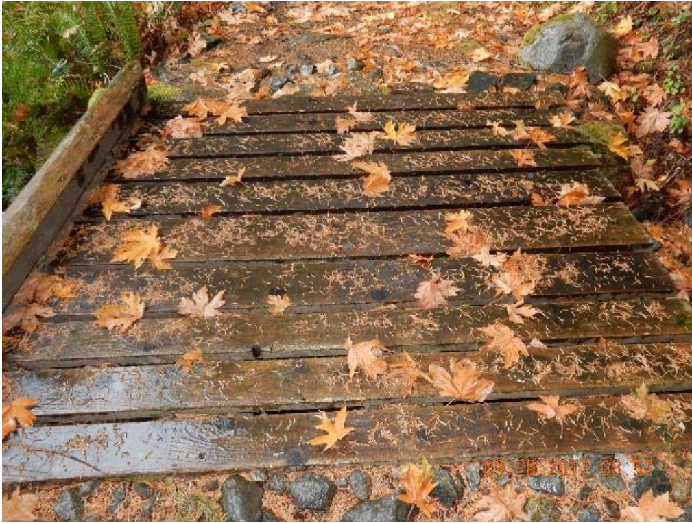
P03 – Overall decking, suggest adding anti-slip pad (DSCN9896.jpg)
