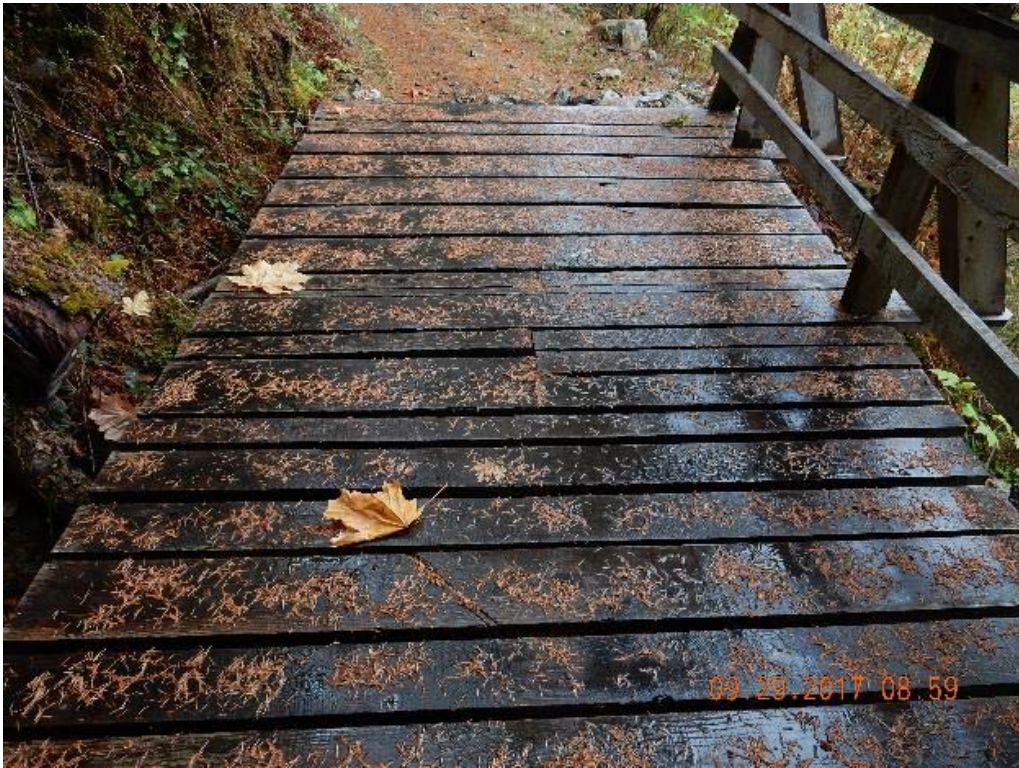
P03 – Overall decking, suggest adding anti-slip pad (DSCN9907.jpg)
