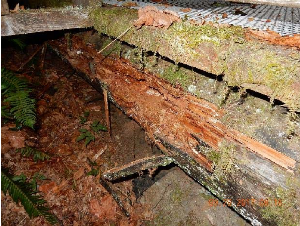
P11 – Northwest corner of the bridge, log is breaking apart (DSCN9859.jpg)
