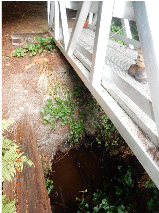
P11 – North embankment, erosion was noticed, needs to be monitored (DSCN0075.jpg)
