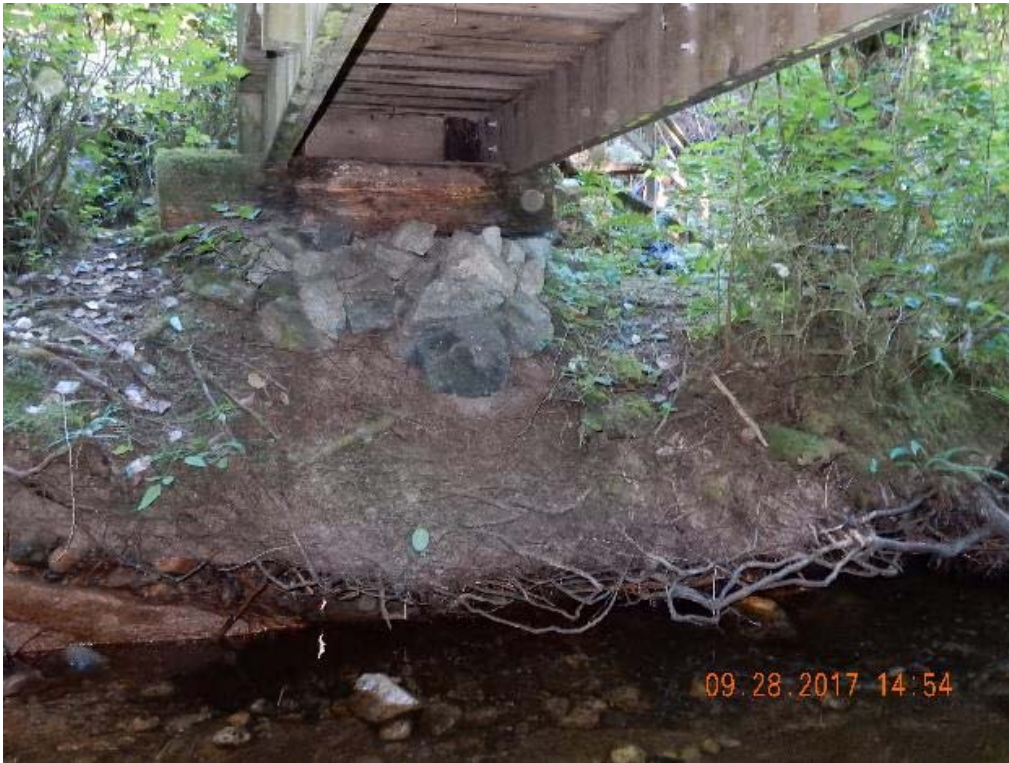
P13 – West span pier 2, erosion was noticed (DSCN9635.jpg)
