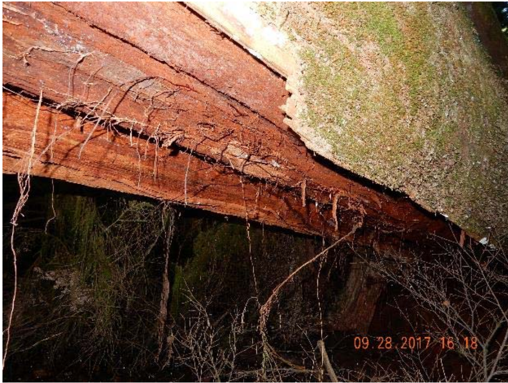
P07 – Under side of the bridge (erosion noticed) (DSCN9700.jpg)
