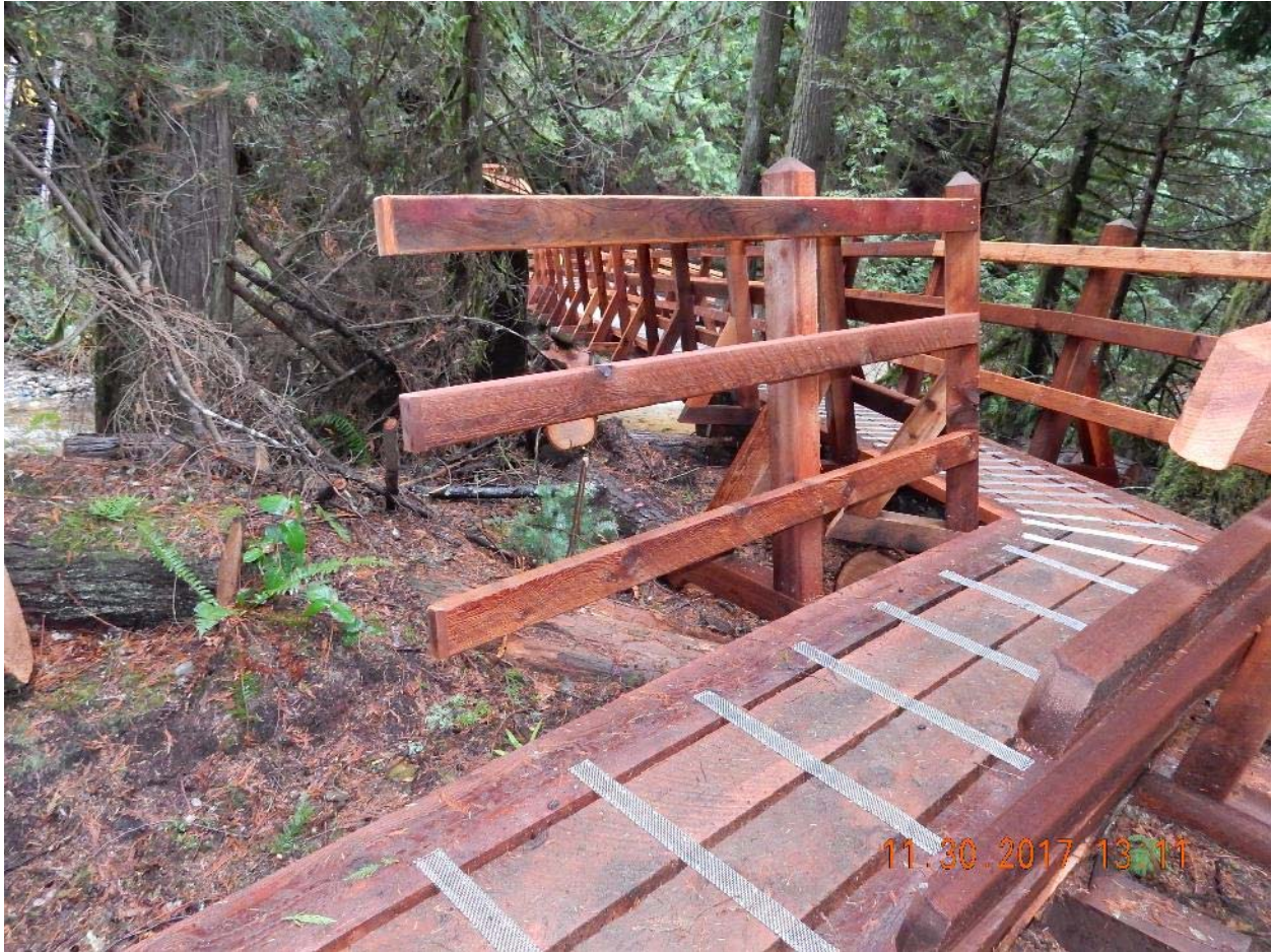
P12 – Railing extending past end post by four feet (DSCN0691.jpg)
