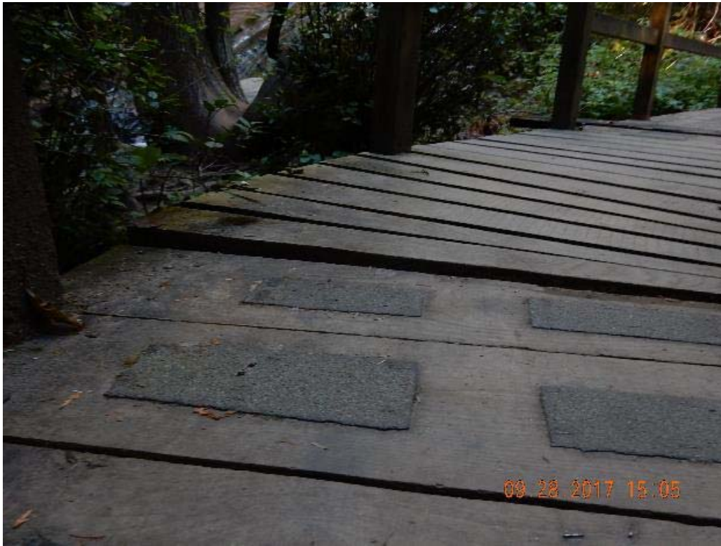
P25 – Right above west span pier 2, starting to settle. (DSCN9652.jpg)
