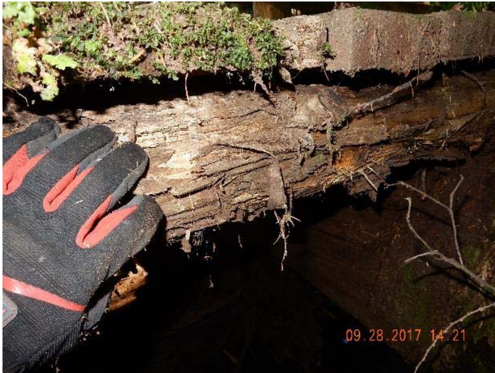
P17 – Pier between west and middle span. Typical deterioration was noticed, suggest having all bridges re-inspected in the next one or two years (DSCN9594.jpg)
