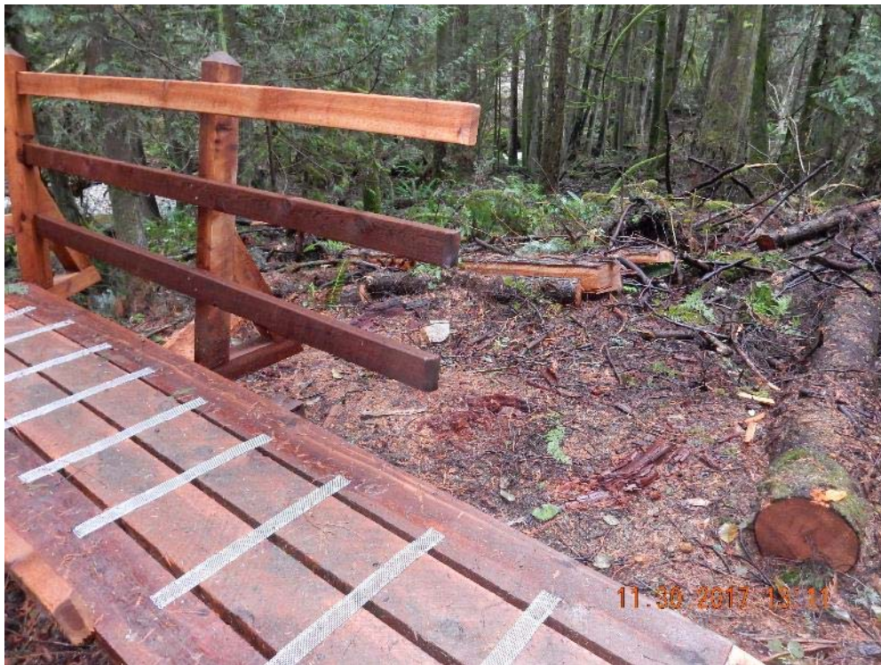
P11 – Railing extending past end post by four feet (DSCN0690.jpg)
