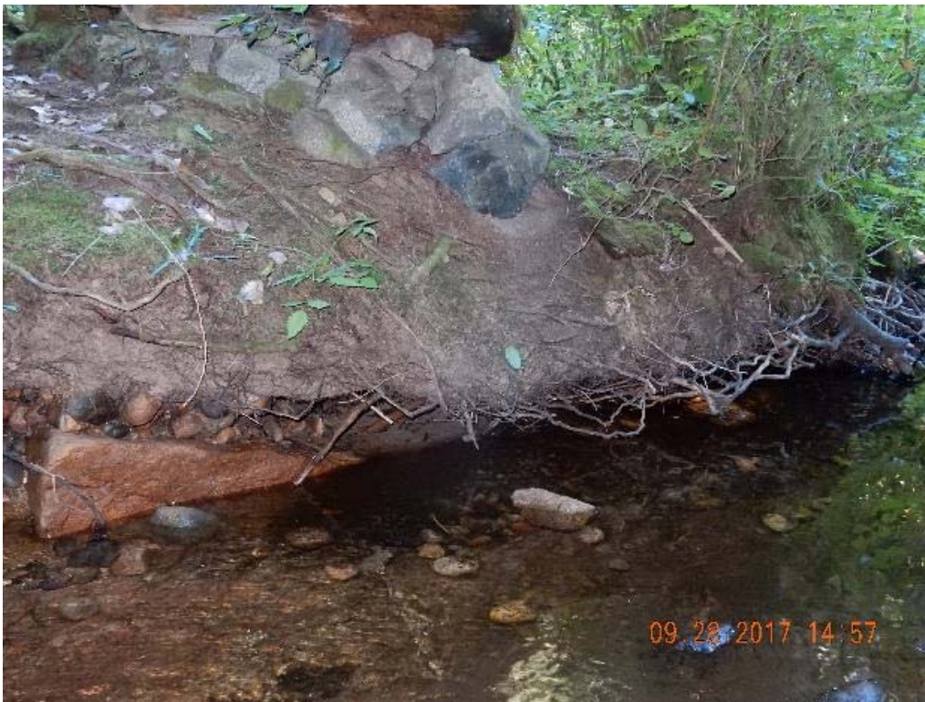
P16 – West span pier 2 (detail view), erosion noticed (DSCN9640.jpg)
