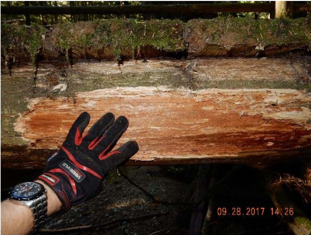
P22 – Exterior bark layer of log beam was pulled off, but the condition is generally ok (DSCN9600.jpg)
