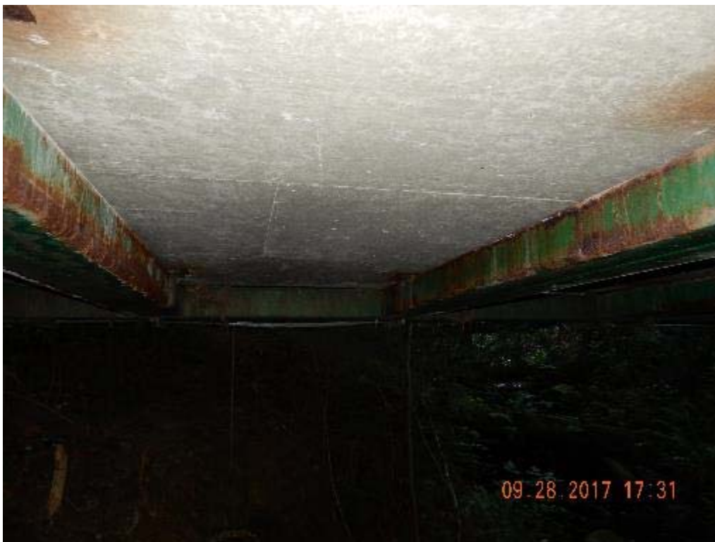
P12 – Under side of the bridge, floor beam and concrete deck (DSCN9814.jpg)
