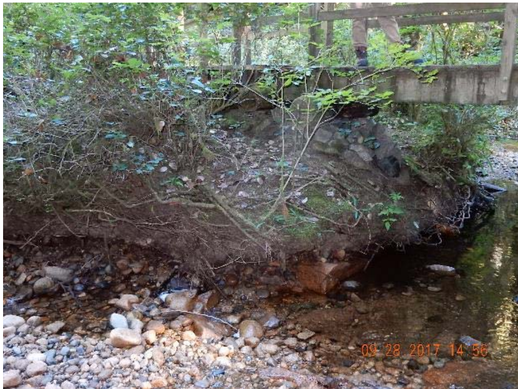
P14 – West span pier 2, erosion was noticed (DSCN9638.jpg)
