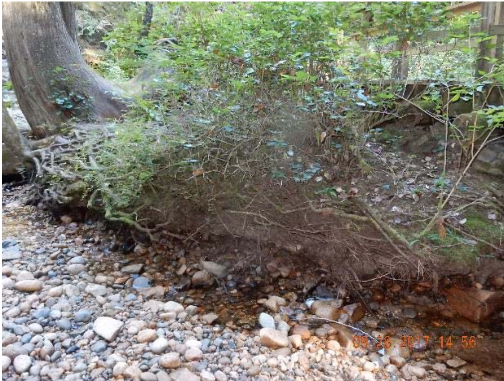
P15 – West span pier 2, erosion was noticed (DSCN9637.jpg)
