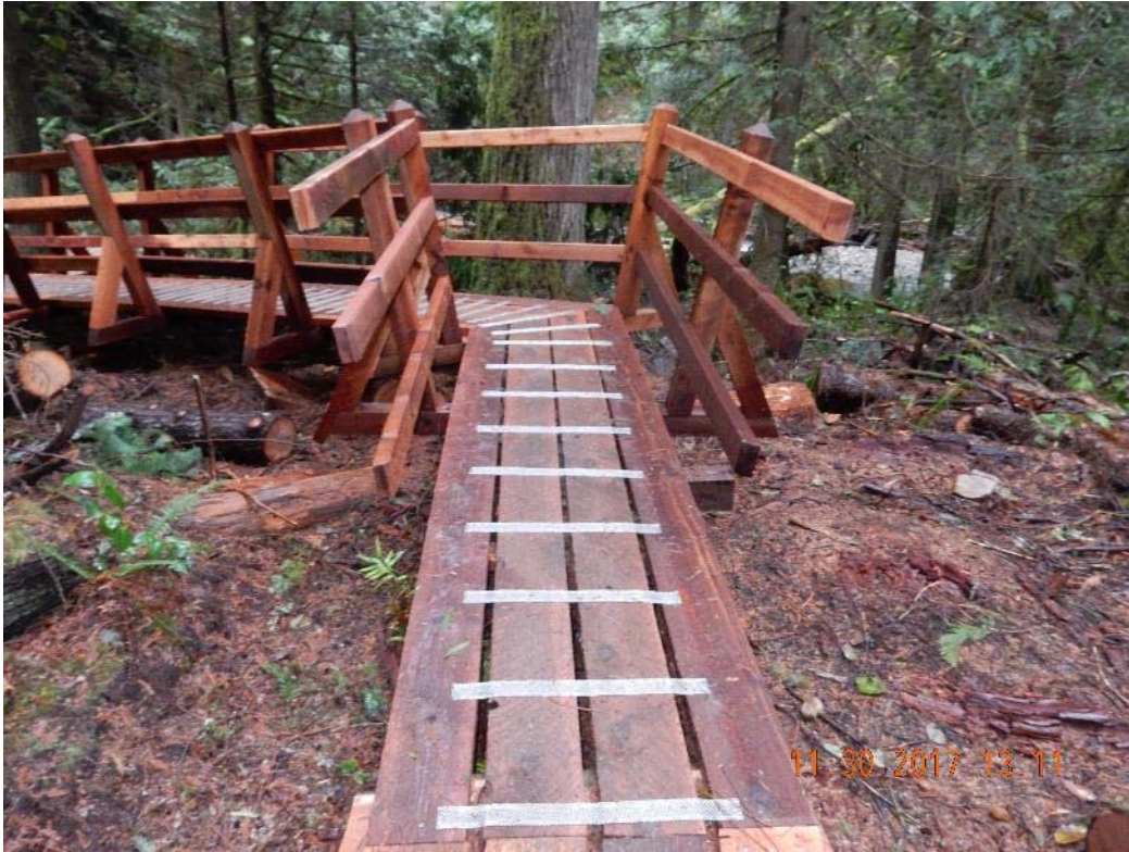
P10 – West Abutment with end railings extending past end post by four feet (DSCN0688.jpg)
