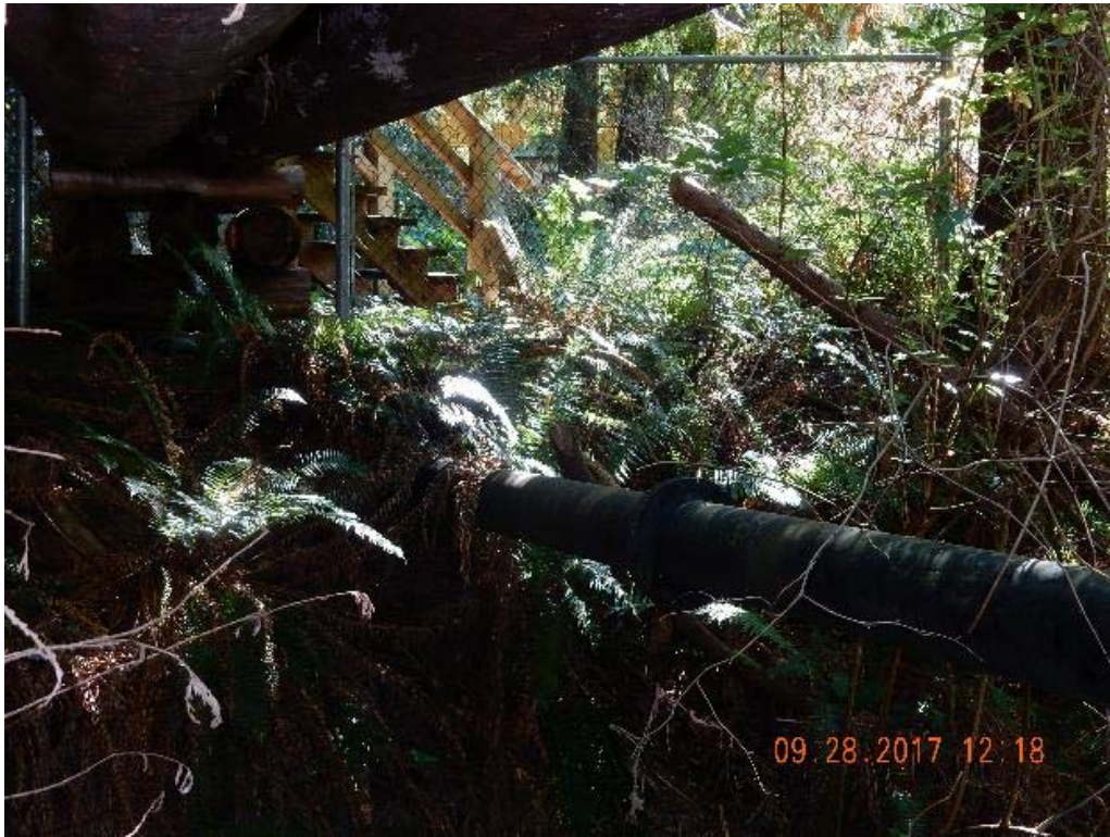
P11 – Utility pipe line to the west side of the bridge (DSCN9535.jpg)
