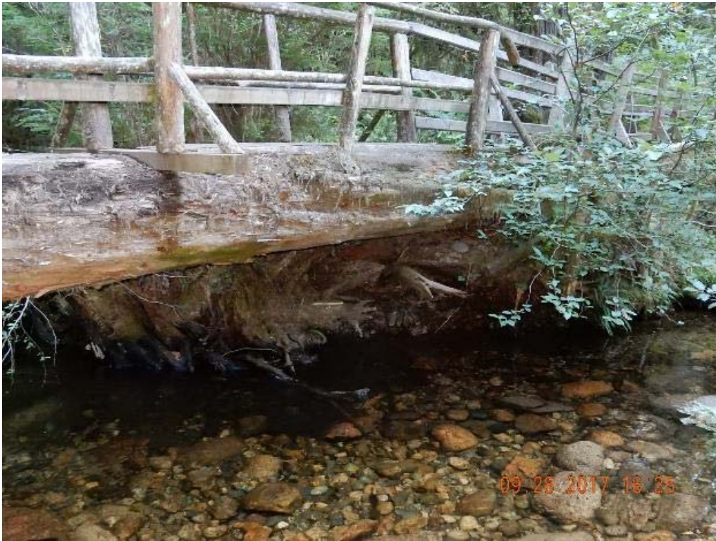
P27 – East abutment of the main span, erosion at embankment was noticed. Suggest putting six or more gabion baskets (DSCN9729.jpg)
