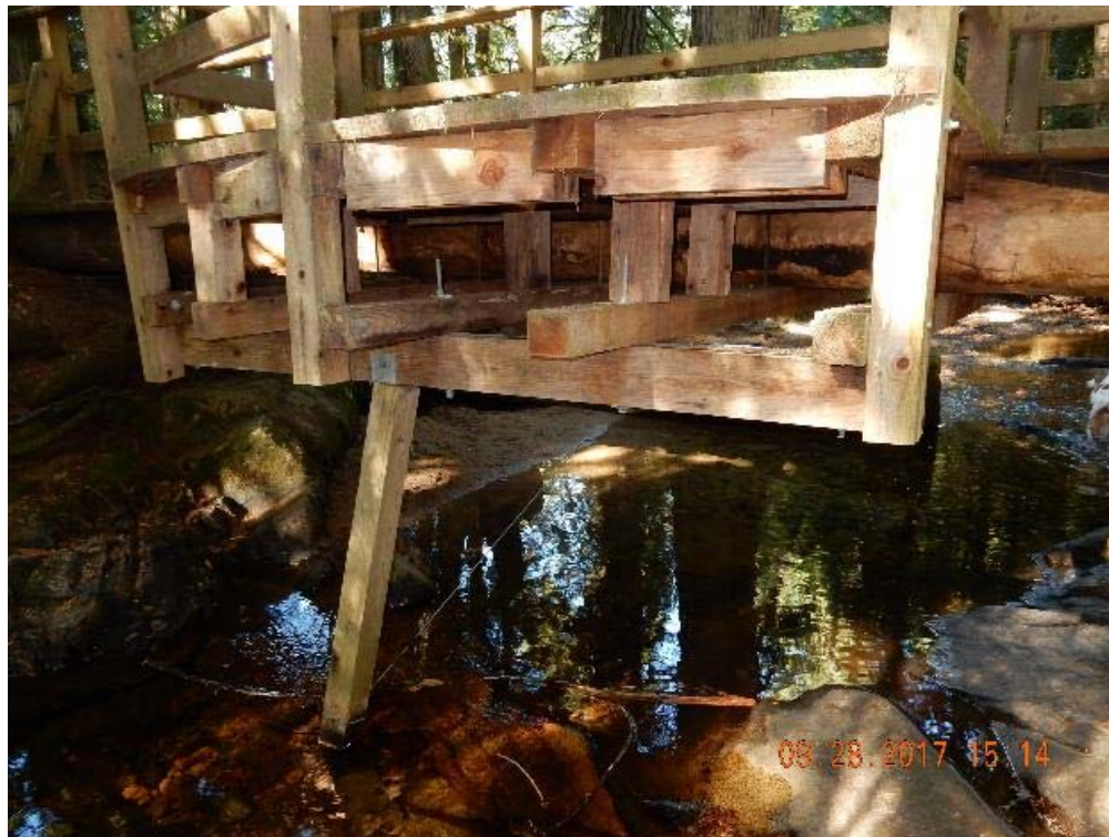
P16 – Cantilever viewing deck supported by one 4" x 4" pole and pulled by cable. Consider adding two more supports at both corners of the viewing deck. (DSCN9674.jpg)
