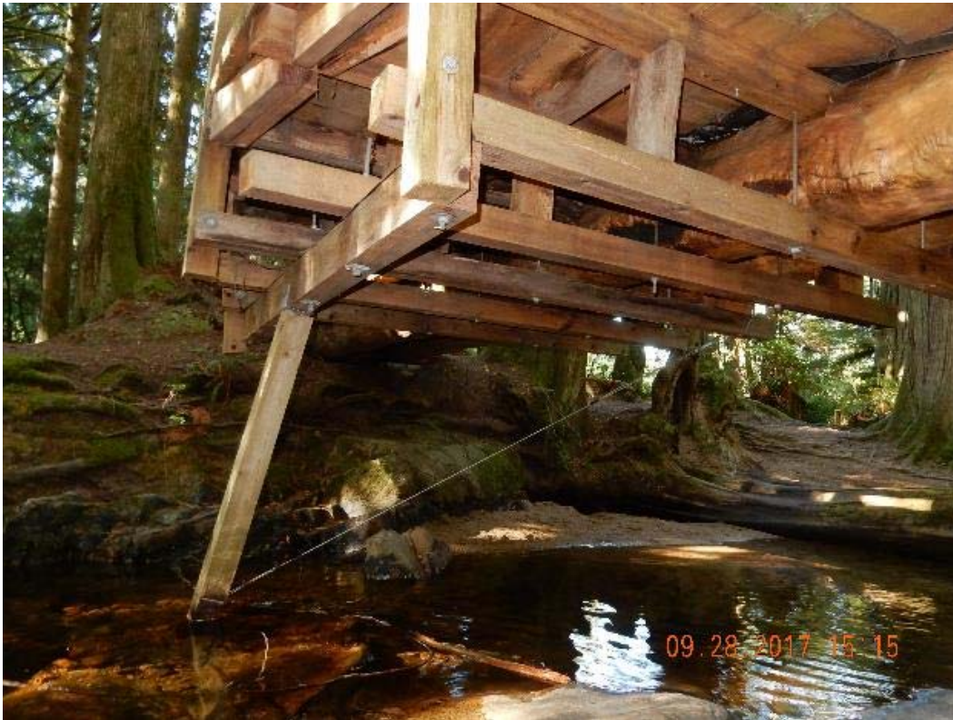
P17 – Cantilever viewing deck supported by one 4" x 4" pole and pulled by cable. Consider adding two more supports at both corners of the viewing deck. (DSCN9677.jpg)
