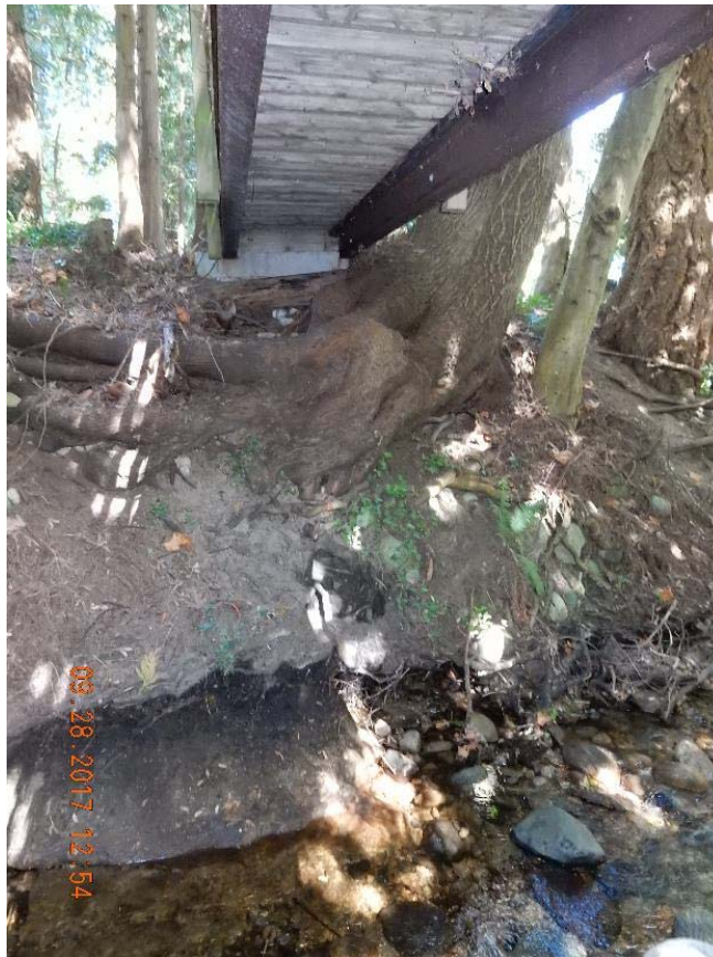
P10 – North embankment. Erosion noticed. Suggest riprap using existing rocks. (DSCN9571.jpg)
