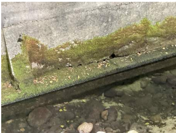
Crack in revetment wall upstream of bridge crossing
