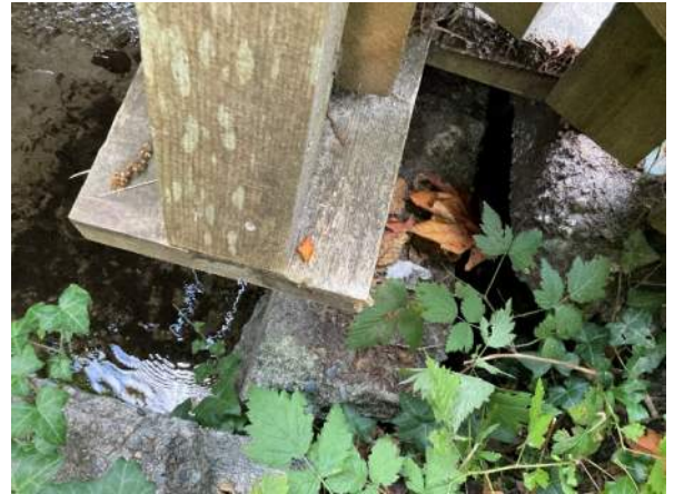
Erosion behind North abutment
