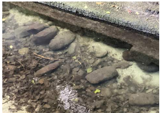
Undermining at revetement wall
