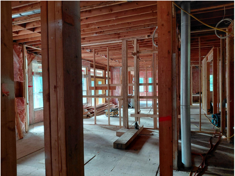
Existing main floor reconfigured for four additional hospice suites, nursing station, family gathering areas.
