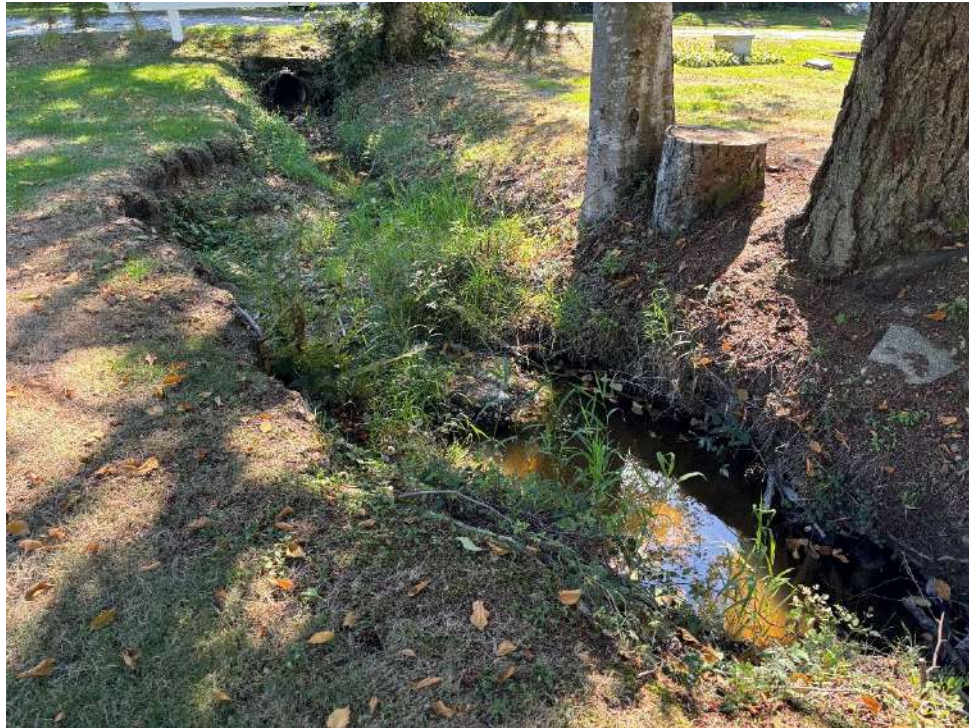
Photo 17: Erosion along west bank of Cornwallis Creek (same as Photo 16)
