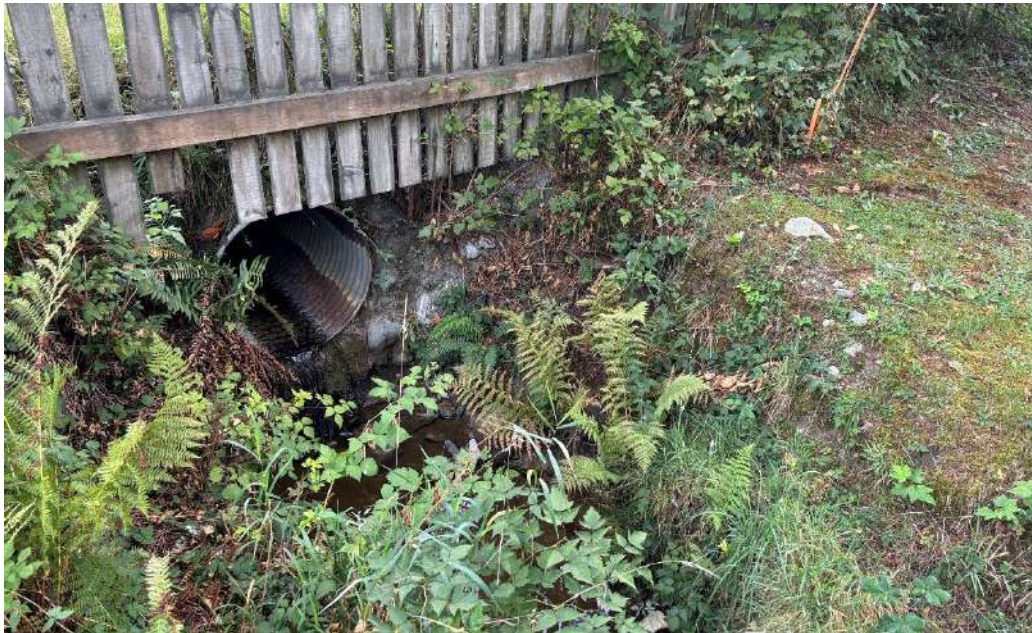
Photo 14: 914 mm (36 in) corrugated steel culvert at upstream end of Cornwallis Creek tributary.
