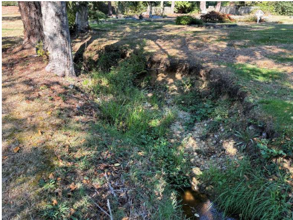
Photo 16: Erosion along west bank of Cornwallis Creek.
