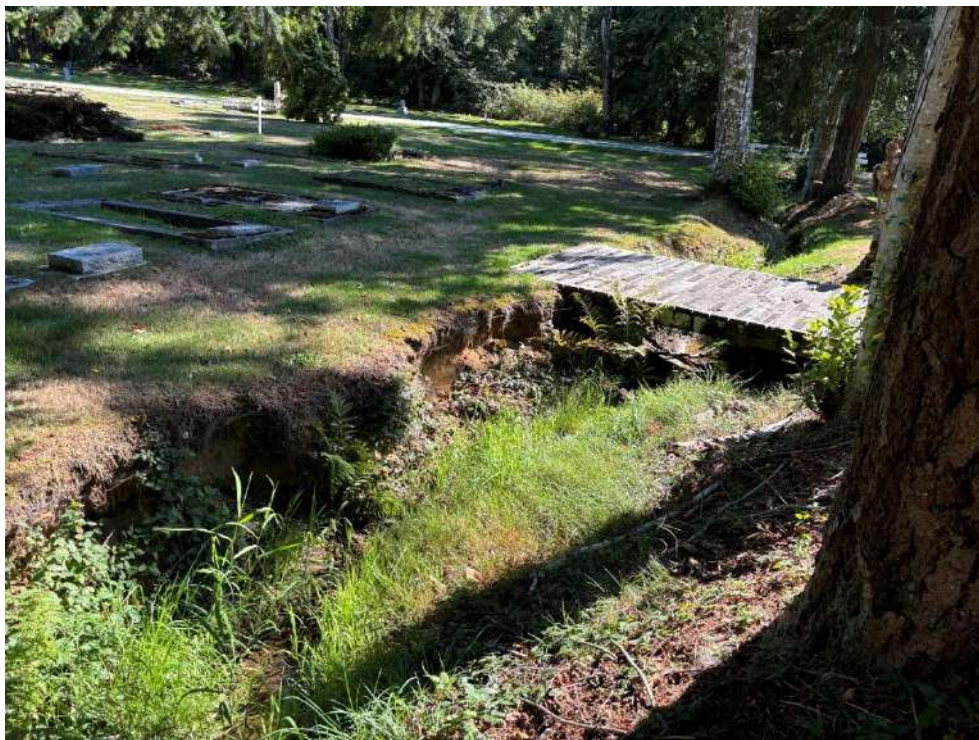
Photo 18: Erosion along west bank of Cornwallis Creek.
