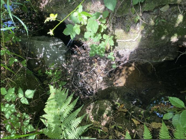
Photo 21 Small debris jam causing water in the Lower Road ditch to go subsurface in Area 1.
