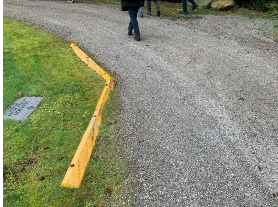
Figure 24: Existing curbing. Opportunity to enhance the cemetery appearance with asphalted driveways and concrete curbing.
